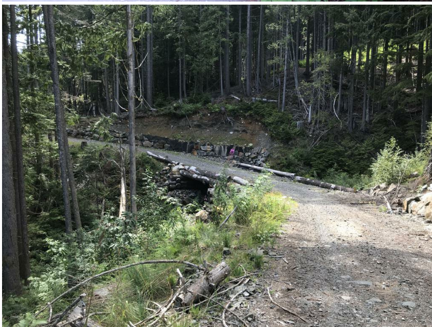
FIGURE 6.9 View of the Sechelt Roberts FSR (7575 Br 23) crossing of a tributary to Chaster Creek at an elevation of 620 m. This example shows a retaining wall that was constructed to stabilize the cutslope and minimize sediment delivery to the stream below. Photo IMG_3093 (Placemark 36), August 24, 2020.
